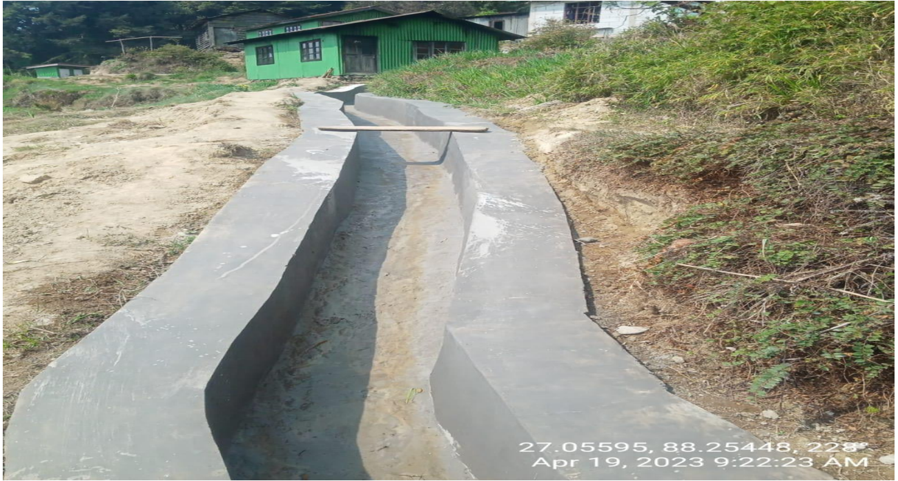
Construction of Catch Water Drain under RAMAM at Namla Forest Village, under Kurseong Soil Conservation Division
